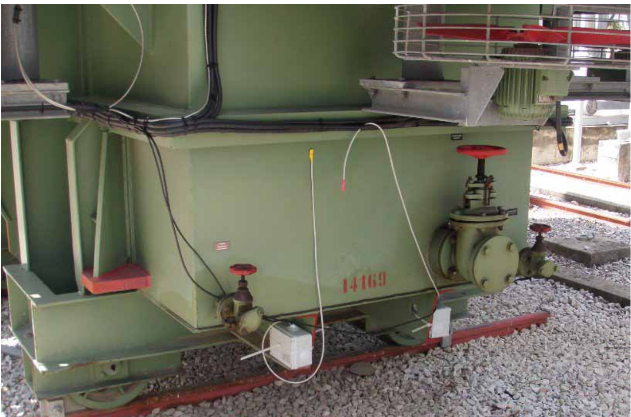
Figure 26. Sensor nodes running the secure microkernel at the EDP substation.
