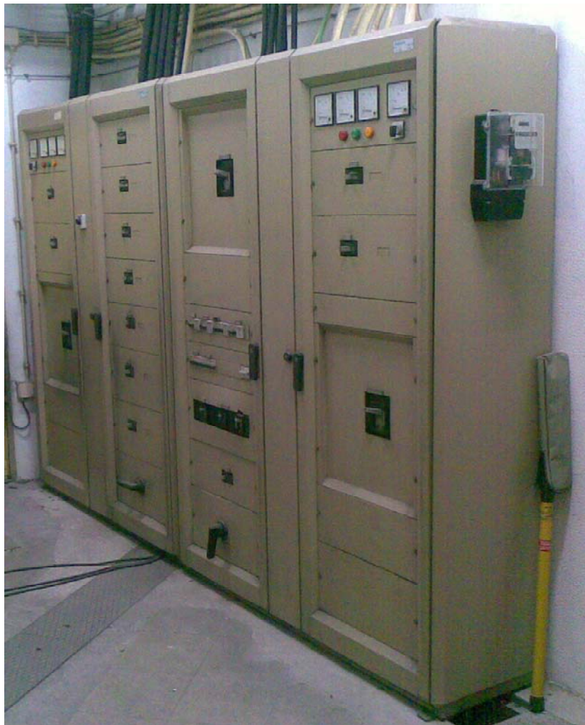
Figure 14: MV/LV power station main switch board.
