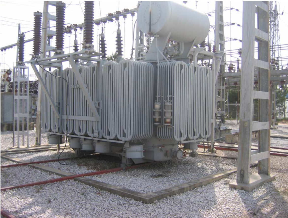
Figure 5: High-Voltage Power Transformer
